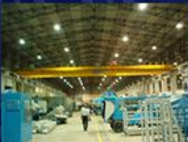
Universal Const. Mech. Ltd - Indoor & Outdoor Industrial work with 22KV HT work.
