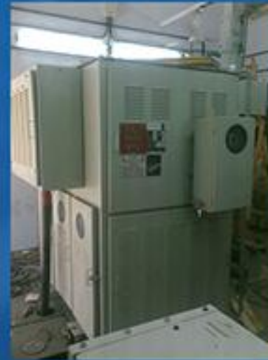
Dry Type Transformer Indoor.
