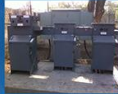
C. Railway ,Solapur -11KV, OD Substation (OSF Unit, HT M. Kiosk, LT Panel, Transformer etc.)
