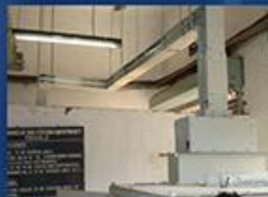
LT compact busduct at BSNL at Goa.
