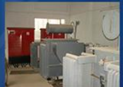
22KV Indoor Substation
