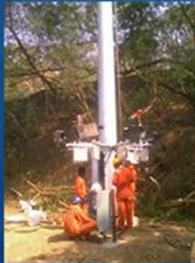
ONGC - 30Mtr. FLP, High Masts with FLP Panels.
