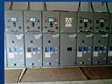
22KV, VCB Panel
