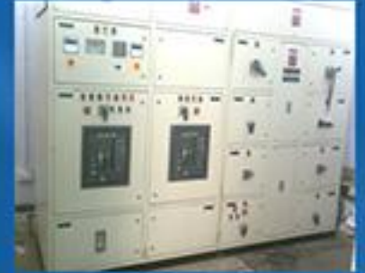
Main LT Indoor Panel
