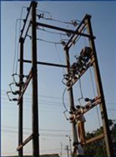
11kv Outdoor Substation For Cwc At Amravat.
