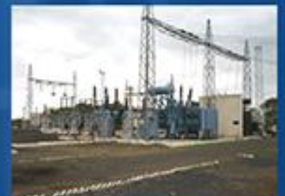
MSEDCL , Latur substation
