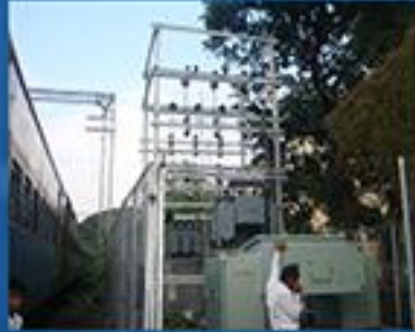
C.Railway -DWS, Pune - 11KV Kiosk with outdoor Substation.
