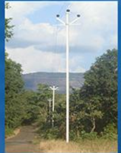
Tops Security Ltd -karjat - 22kv Ht & 22kv Substation
